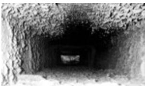
Before duct cleaning
