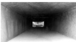
After duct cleaning
